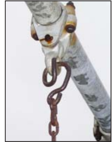
Open "S" hooks and protruding bolts present many hazards on the playground.
